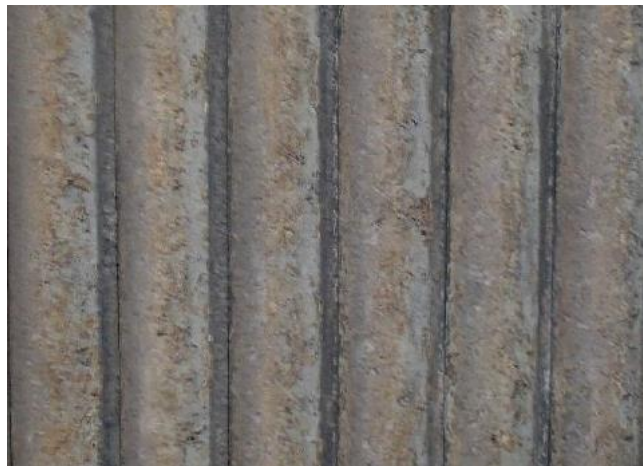
Corroding boiler tubes, Drax, 2018
